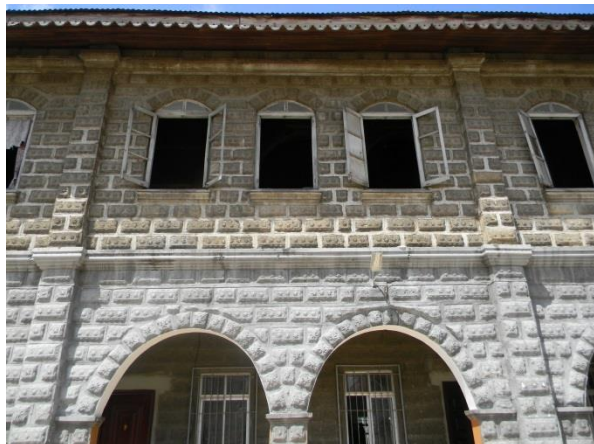
Figure 23: Use of arched windows and CMUs to replicate cut stone Source: Author (2022)
